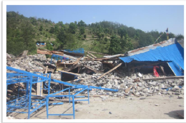
The dormitory building after the 2015 earthquake
