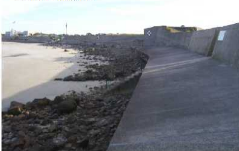
Plate 6.11. Build up of shingle at the southern end of DU2
